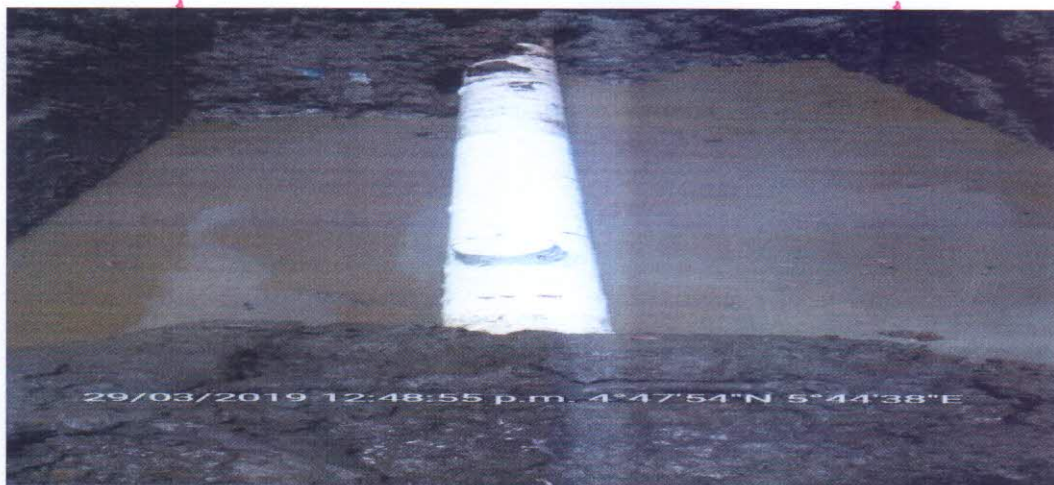
Picture showing spill point ,cause of spill and point after repair.
